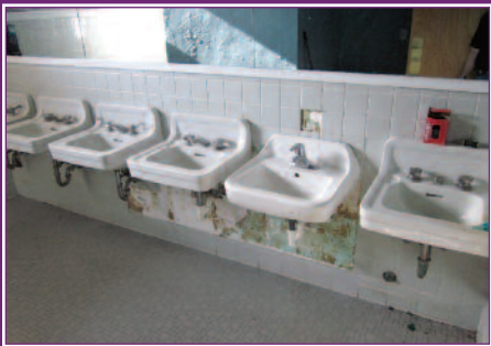
The plumbing for the sinks of the freshman bathroom has been a constant issue, and after years of use, a majority of the wall tile is missing under the sinks.
