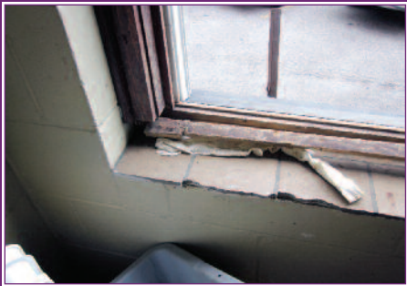
Due to the use of a window air conditioner, the sill of this window in the kitchen is gone.
