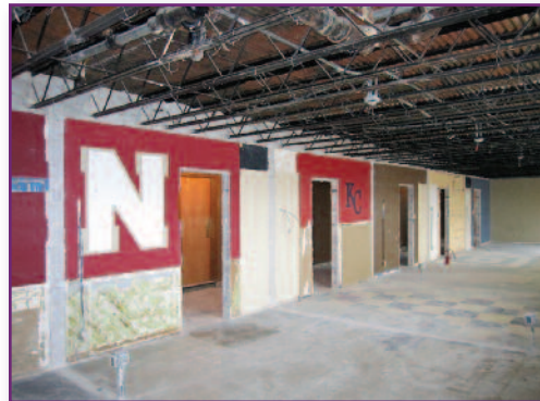
All of the walls and ceilings in Sophomore Hall have been removed to make room for new suite-style units, fire sprinklers, and central heat and air conditioning.
